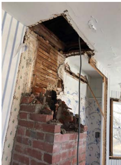
A small second floor bedroom fireplace. It was unusable, but lovely to imagine its warmth and comfort in the 1800's in an uninsulated house
